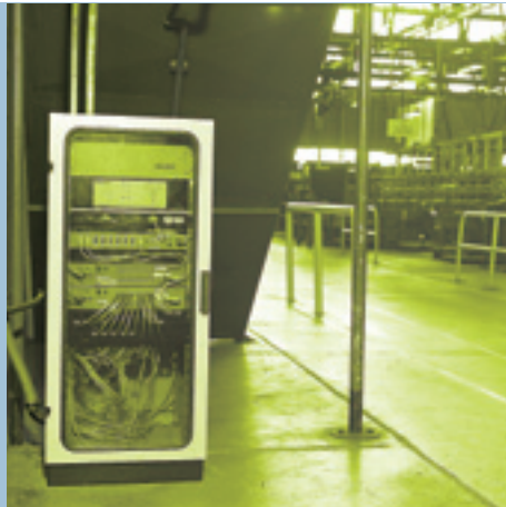
Industrial Cabinet in a factory environment.
